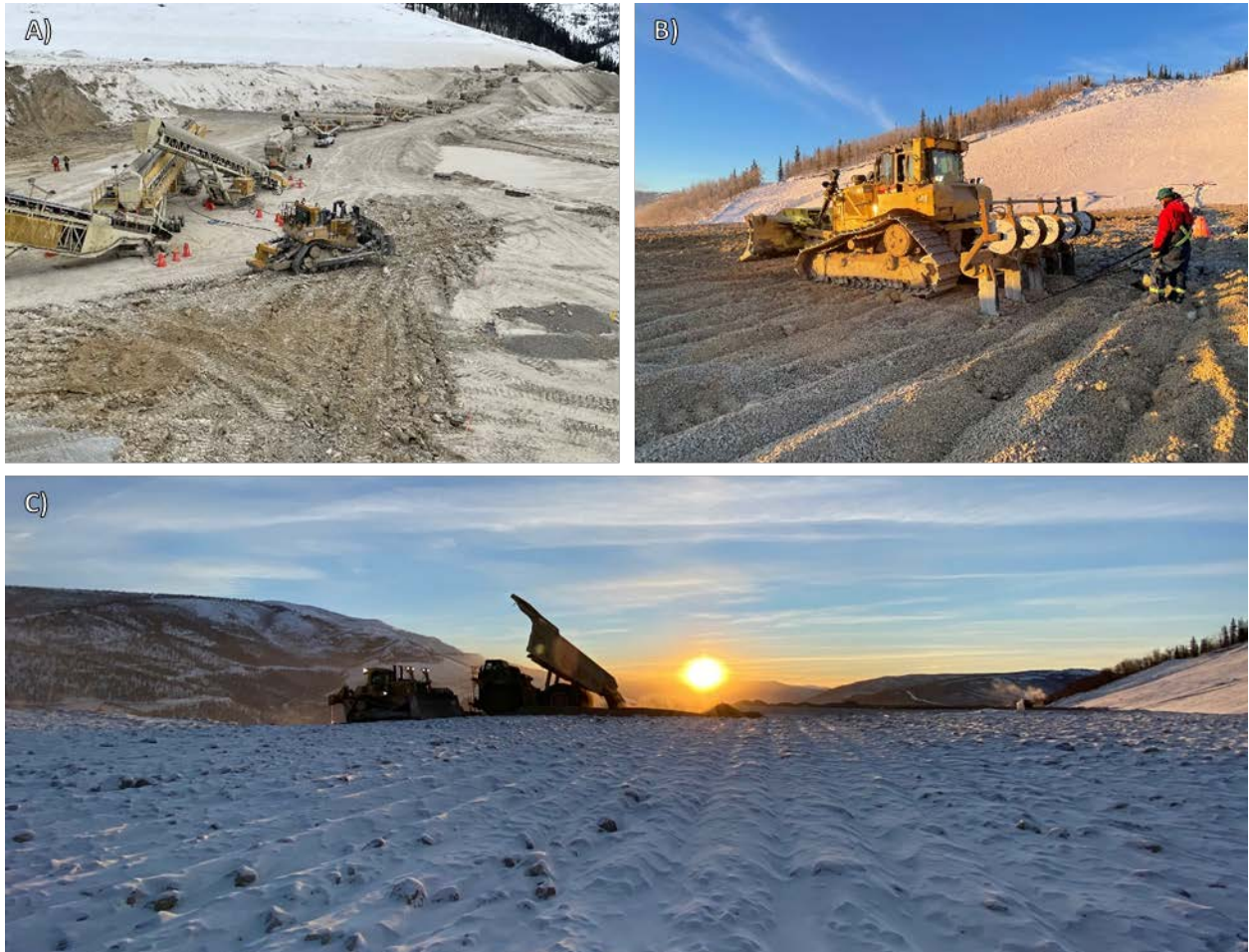
Figure 4: Leaching operations at Victoria Gold Corp. A) Cross ripping ahead of advancing stacking B) Installation of buried drip lines C) Leaching area
