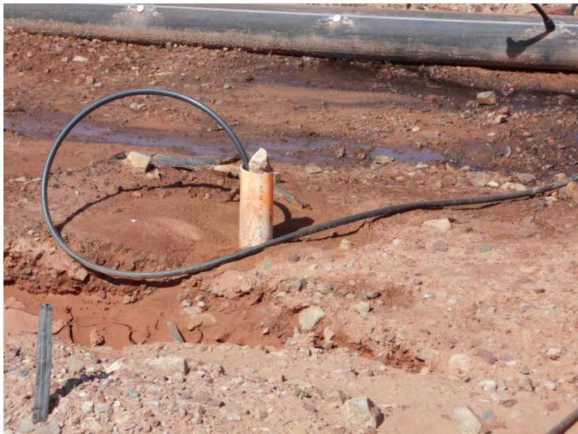
Figure 1: Gravity or deep raffinate well installed atop a heap leach pad
